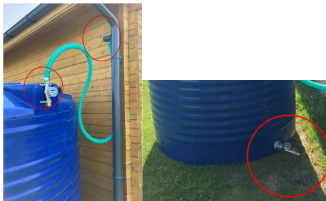
Figure 1. Rainwater harvesting tank in the analyzed farm
